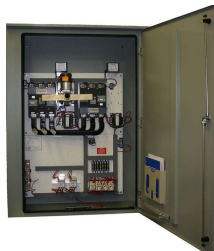
Florida Power and Light ATS (Electro Mechanical)
